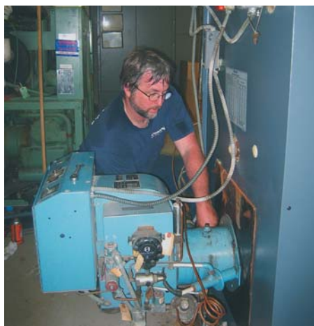
Brian Crispin tunes up the boiler at Slack Inc.
